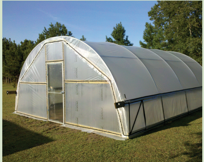
Construction of the 600 square foot demonstration high tunnel was completed in eight hours.
