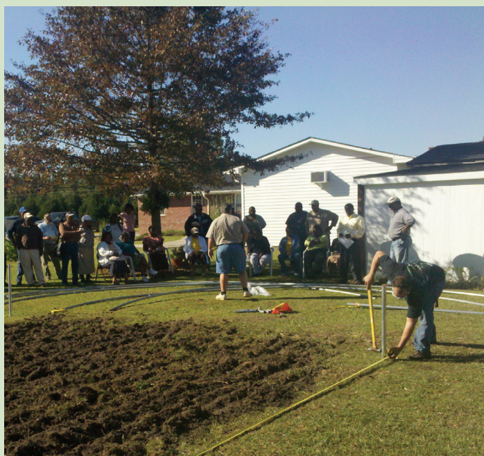
Farmers in Williamsburg County helped construct a high tunnel. One of the first steps was squaring the base.
